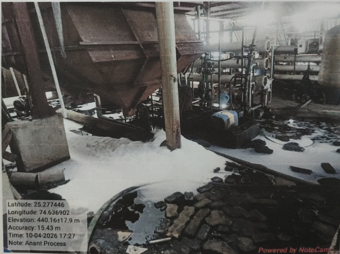
Figure 6. Flexible Pipeline found near effluent accumulated at M/s Anant Syntex Ltd
