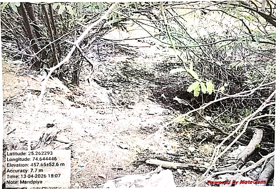
Figure 9. Rectified Nut Bolt arrangement attached with Pipe line at Mandapiya unikt of M/s Anant Syntex Ltd
